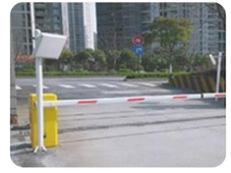
Vehicle Access Control
